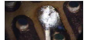
cold (grainy) solder joint
