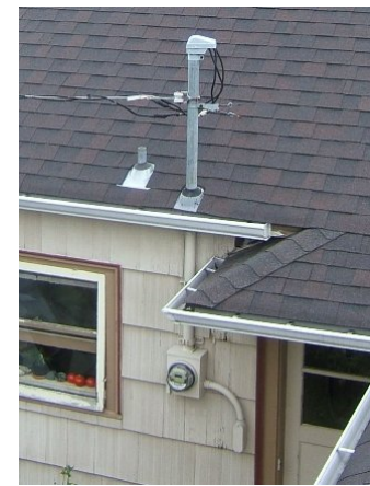
electrical service drop
