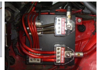
power distribution block with both a
