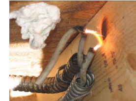
arcing between wires
