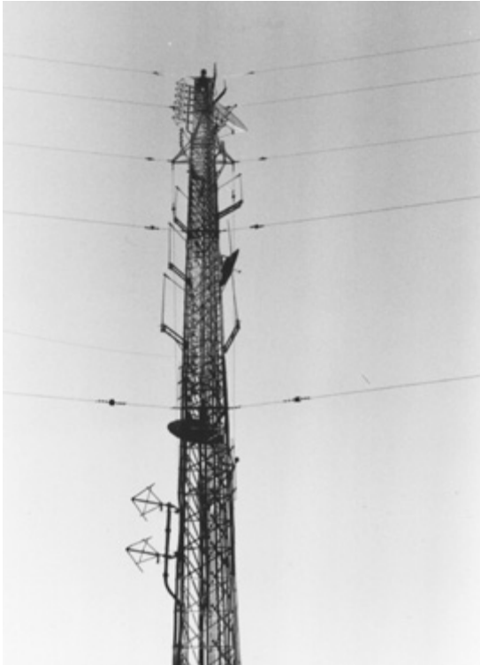
1-1 This AM/FM broadcast antenna tower bristles with two-way antennas.
